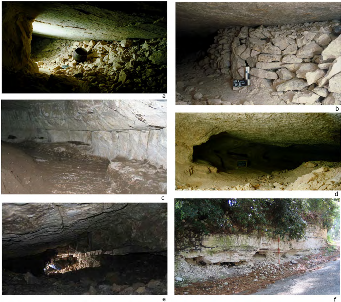
Fig. 3 – Some examples of sub-horizontal mining systems (type A). a, b, d: Defensola A, mine no. 1; c: S. Marco; e: Tagliacantoni; f: Martinetti, mine no. 1.
